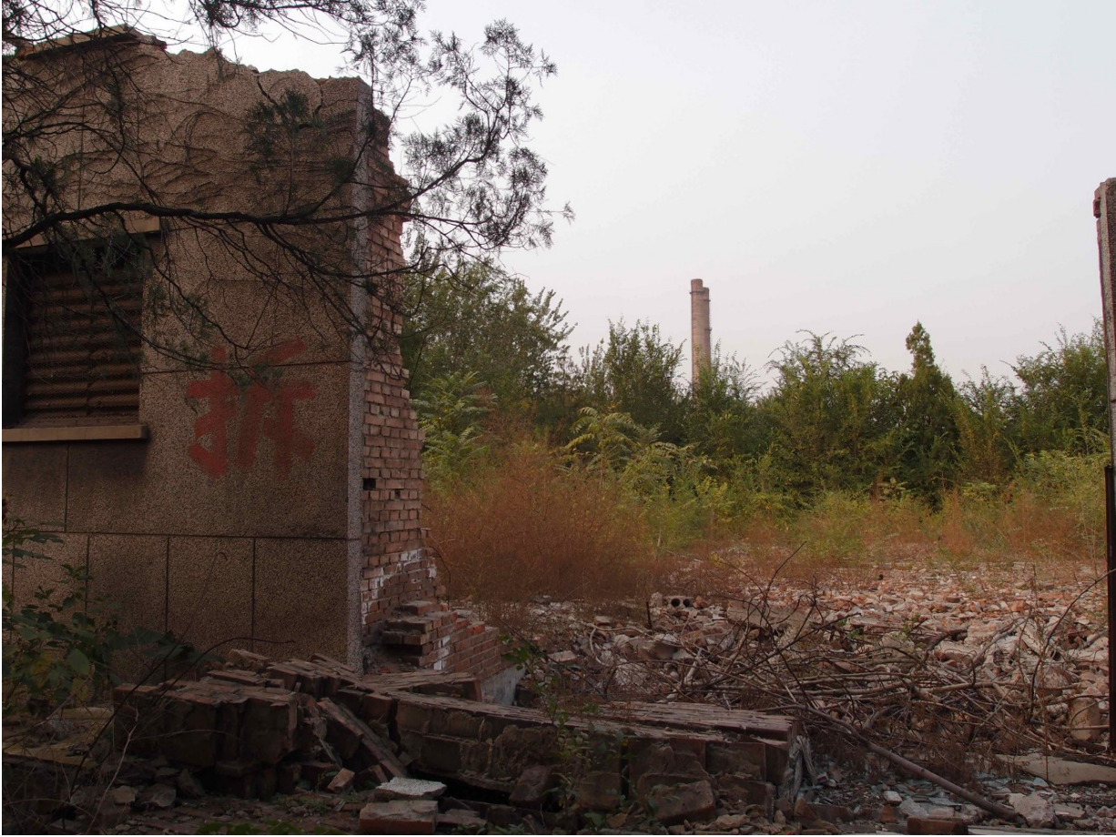
Photo 21. Part of the Shougang industrial complex in the process of being demolished, Beijing, October 2015
